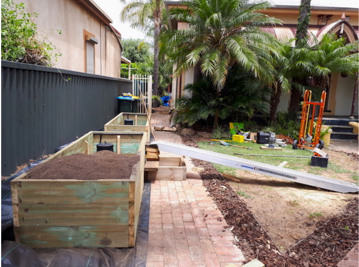
The front bed is half filled with soil and the ramp is placed ready to fill the other half.
