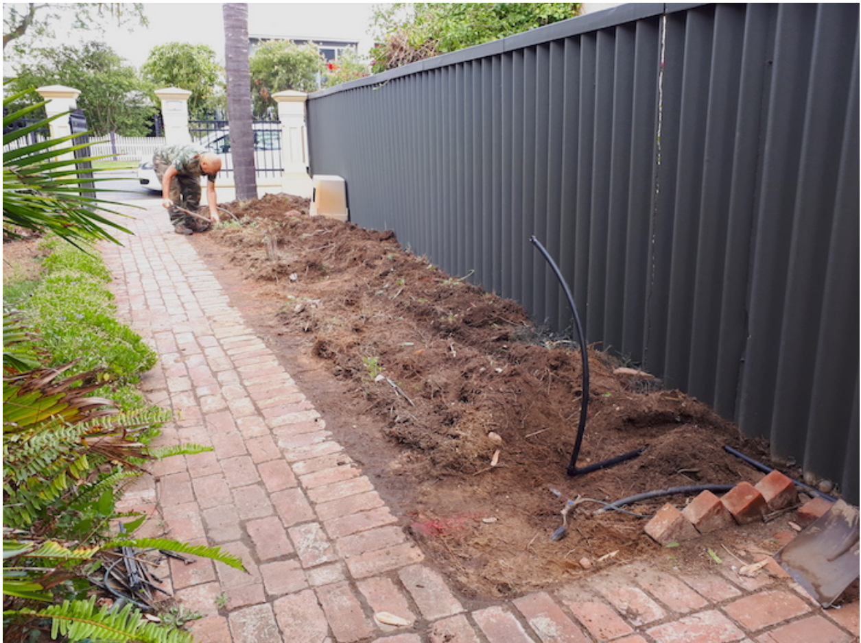
The ground work - digging up tree roots and digging trenches for the irrigation pipes and the garden beds.
